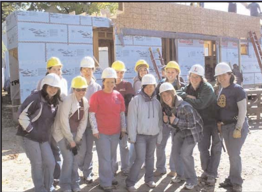
Students in the UMF Rotaract Club committed their time and talents recently at the Auburn Habitat for Humanity building site where they helped to build a home for an area family. (UMF photo)
